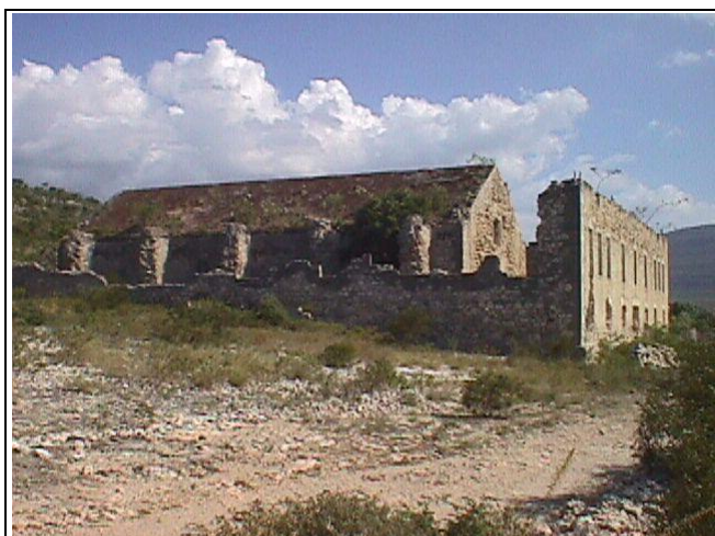
Figure 48 Remnants of a time when Haiti had a functioning State. King Henri Christophe used this building in the early 1800s to make gun powder for one of the largest standing armies in the world. Vie, Katie, Mole Saint Nicholas (See endnote 2, Chapter 1 for brief description of the Kingdom.)
