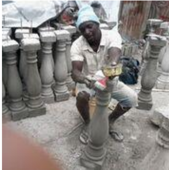
A mason on a Saint-Marc construction site, after participating in the worker survey.
